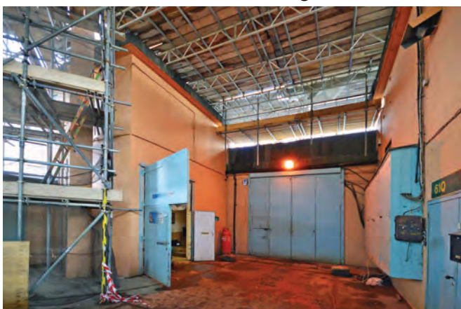
The main entrance doors of Non-nuclear Component Building 61 (the easternmost of the two). Plant rooms flank the entrance, while above, repairs to the roof and to the gantry concrete are in progress
